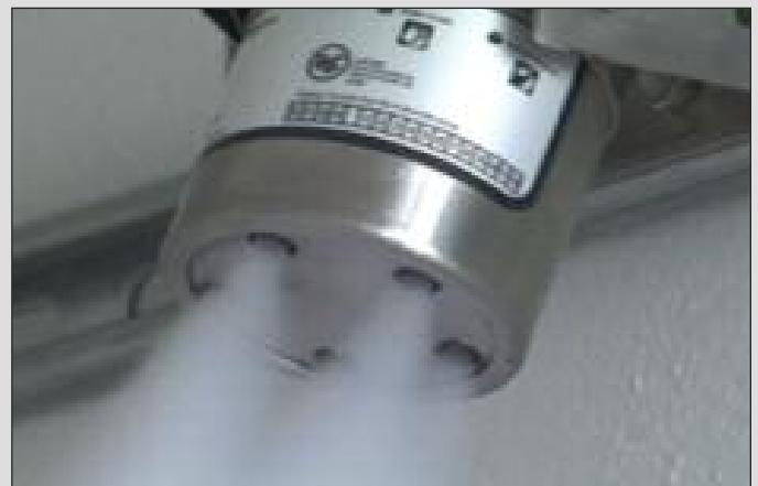
Stat-X® unit discharging.
